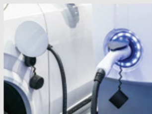
Individual EV charging provision in each car park
